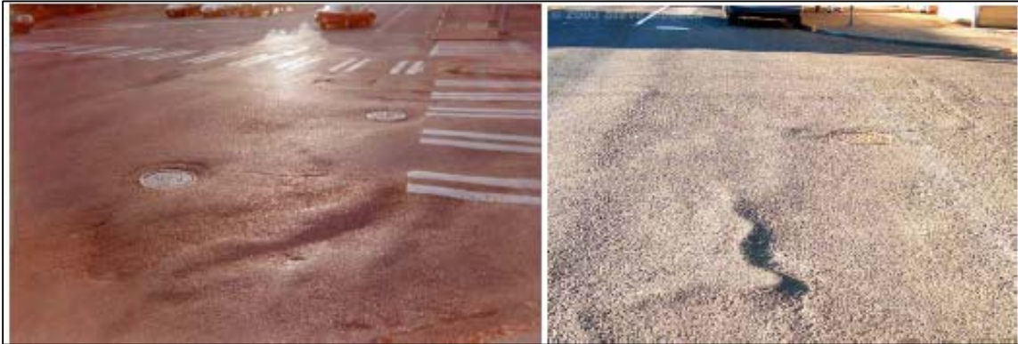
Figure 7: Shoving on Asphalt Pavements.
